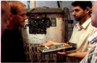
Nautel's Aaron Debaie trains Teracom engineers during commissioning of the NX50-LW transmitter. (Photo by Niels Dreijer)
